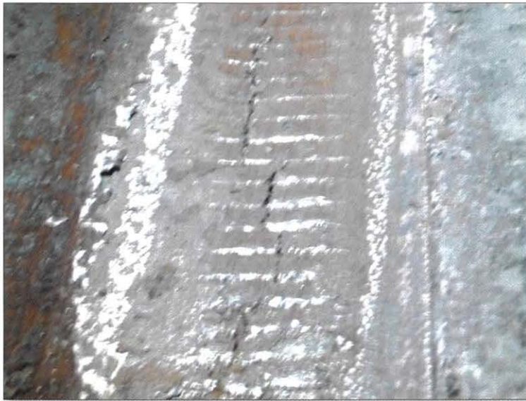
Fig 1 Web surface cracks on beam blank
