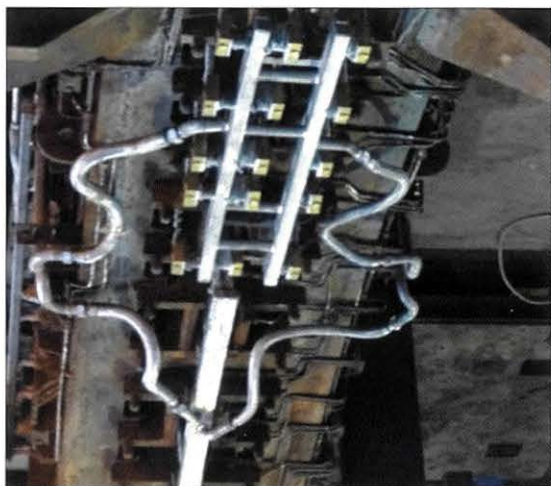
Fig 6 Segments 1 & 2 with new air-mist headers mounted on strand 1 during cold commissioning
